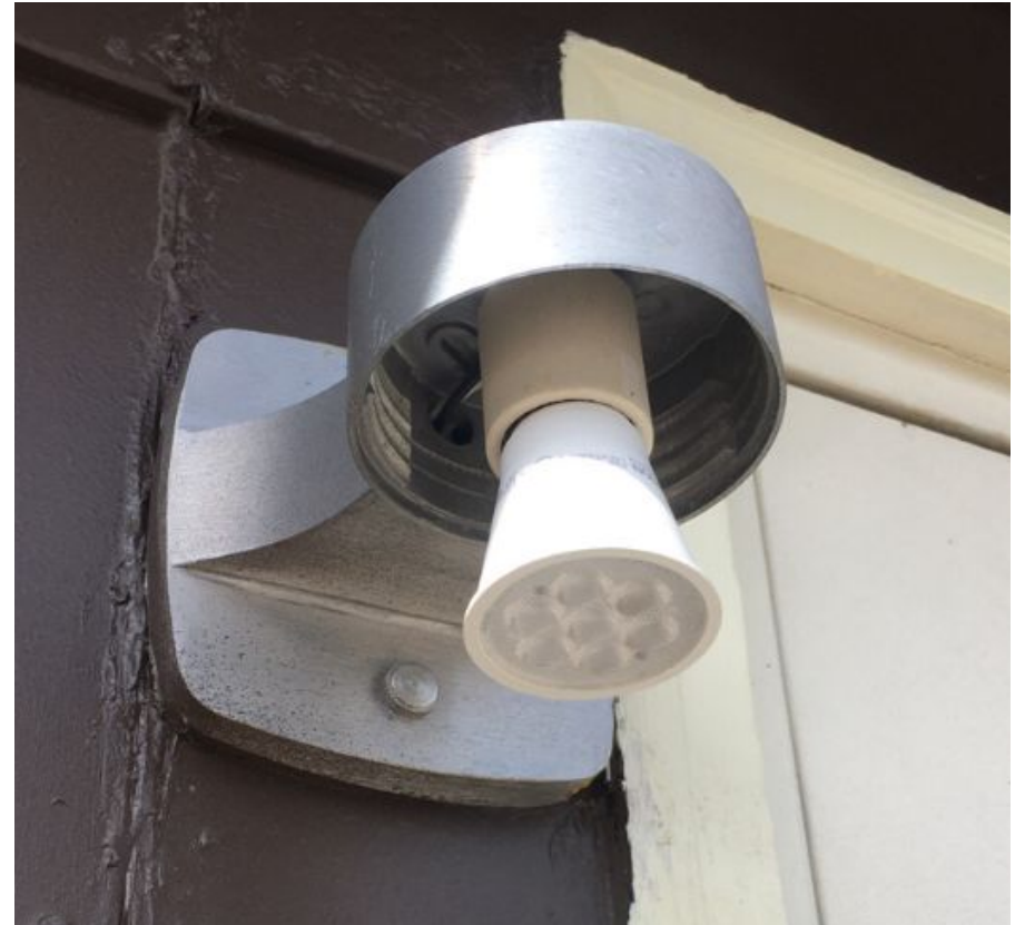
Figure 11. Example of a fully shielded bulb, able to turn a non-compliant lighting fixture into a compliant one. Photo by Christiana Kearns.
