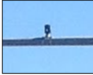
Figure 22. Preemption device placed on traffic signal poles to detect approaching emergency vehicles.
