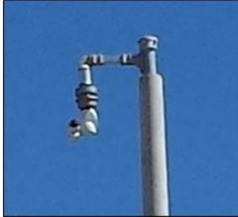
Figure 12. COHU Closed Circuit Television Camera
