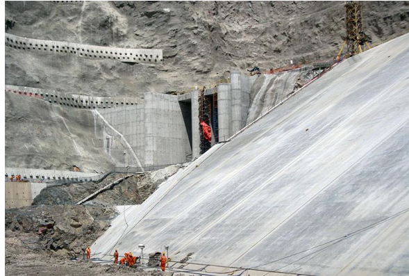
Figure 1: Shown is the dam under construction. Note the smooth surface of the dam created by the cart dragging process.
