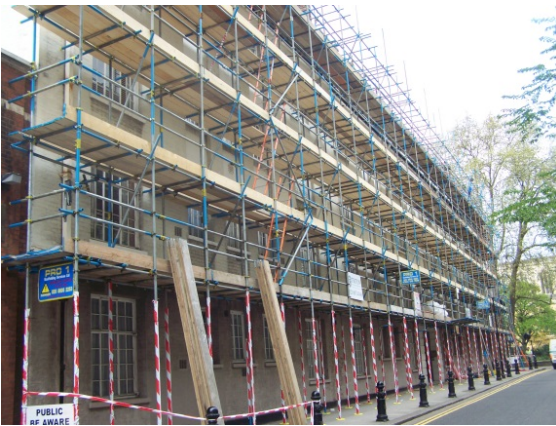
Figure 17 U.S Metal pipe scaffolding (Hunt, 2005)
