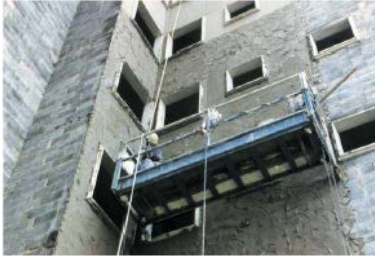
Figure 14 Brazilian System of Suspended Scaffolding (Callegari, 2012)
