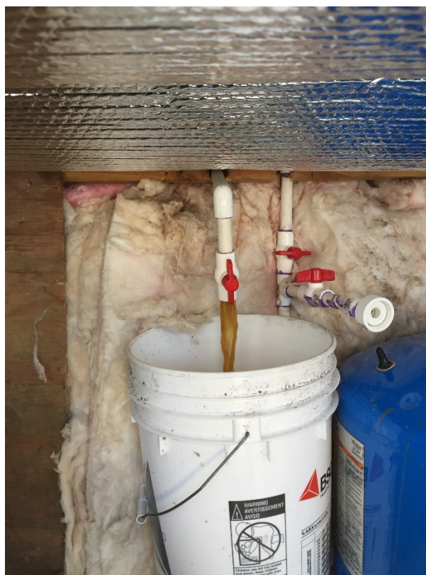
Figure 17: Effluent drainage system
