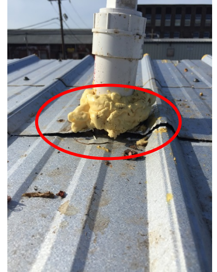
Figure 19: Popped roof from excessive pressure
