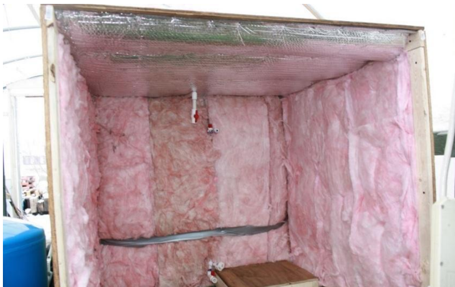
Figure 8: Insulated collection space, Phase 1
