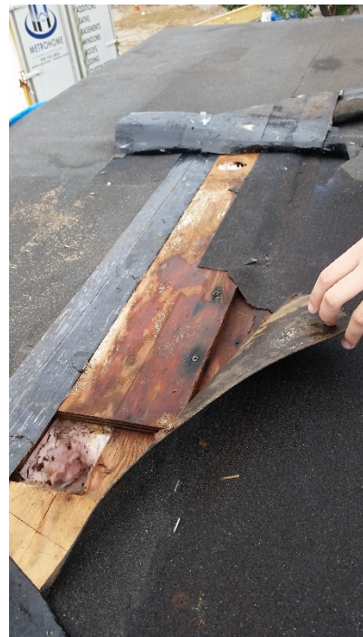
Figure 9: Damaged old roof
