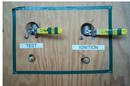
Figure 3-2: Burner control valves
