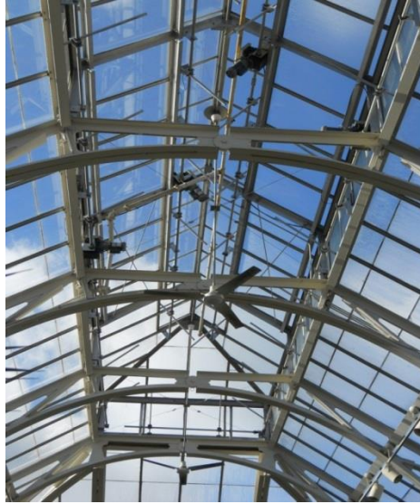
Figure 20: Ceiling fans and motorized vents at Tower Hill Botanic Gardens
