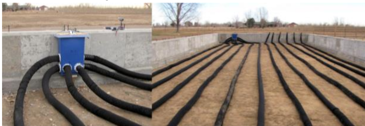
Figure 73: "Two Greenhouse Earth Storage Systems (GETS) installed, vertical rigid R-10 Styrofoam in place. A second R-10 sheet was installed, then horizontal R-10 sloped gently downward 2.5 feet below surface."
