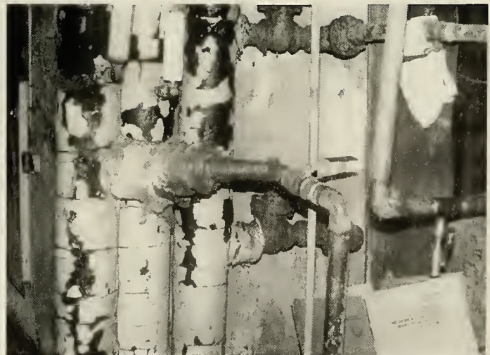
A view of the Pentagon's deteriorating heating and cooling plant.
