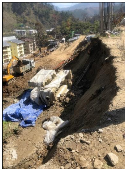
Figure C: Rapid vulnerability assessment on campus (Photo Courtesy: Brainard, 2019).
