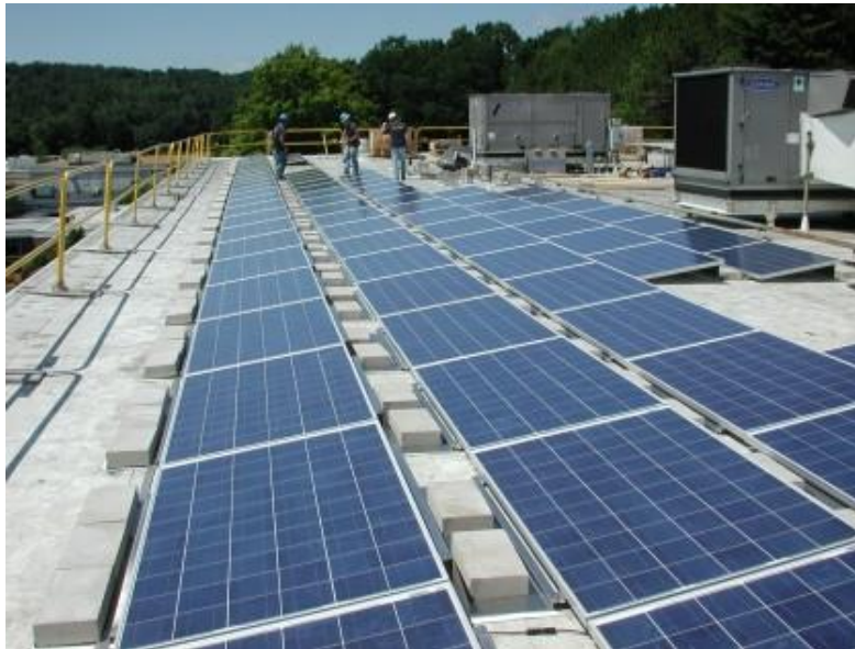
FIGURE 19: TYPICAL SOLAR INSTALLATION BY FUTURE SOLAR SYSTEM LLC [22]
