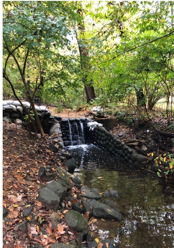
Figure 6: A leaking historical dam in Dumbarton Oaks Park
