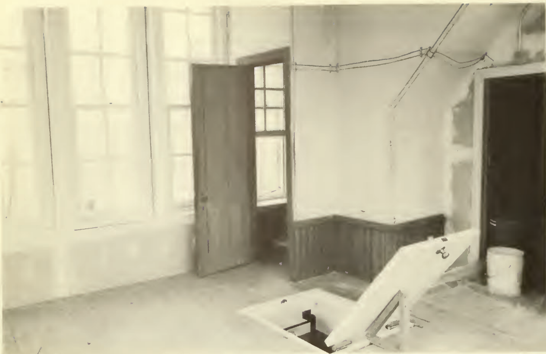
The northwest corner of the tower room, with the stairs leading to the clock and roof, and the site of the graffiti.
