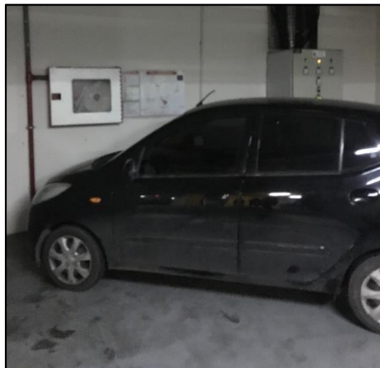
Figure 14: Blocked access to hose reel in Morocco Mall parking garage
