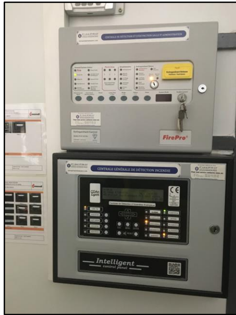
Figure 28: Fire panel in the Mondi administration office
