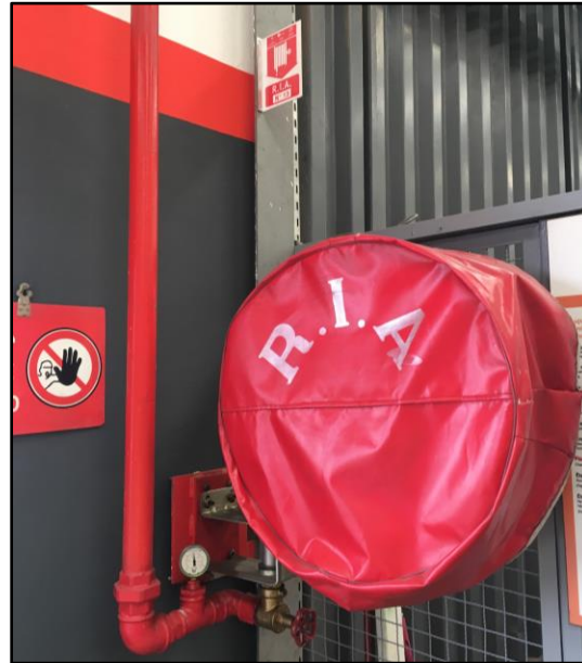
Figure 26: Fire hose in the production area of Mondi Pap Sac Maghreb
