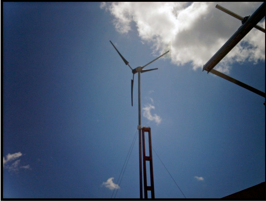
Figure 4- 6: Small wind turbine at the Polytechnic University of Puerto Rico
