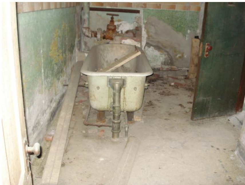
Figure 5. Continuous bath tub remaining at Grafton State Hospital.
