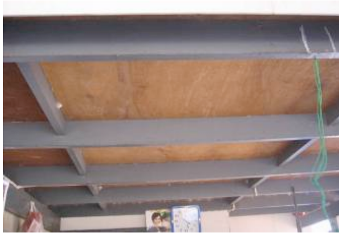
Figure 13: Non-Reinforced Second Story in Ban Tub Nua
