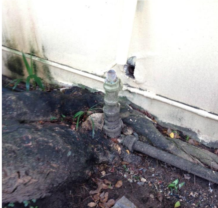
Figure 1. Root Damage to Piping
