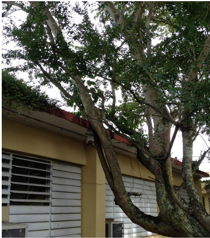
Figure 6. Branch Damage to Roof 3
