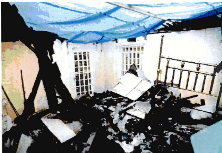
Figure 4.2(a): “Interior Damage”
