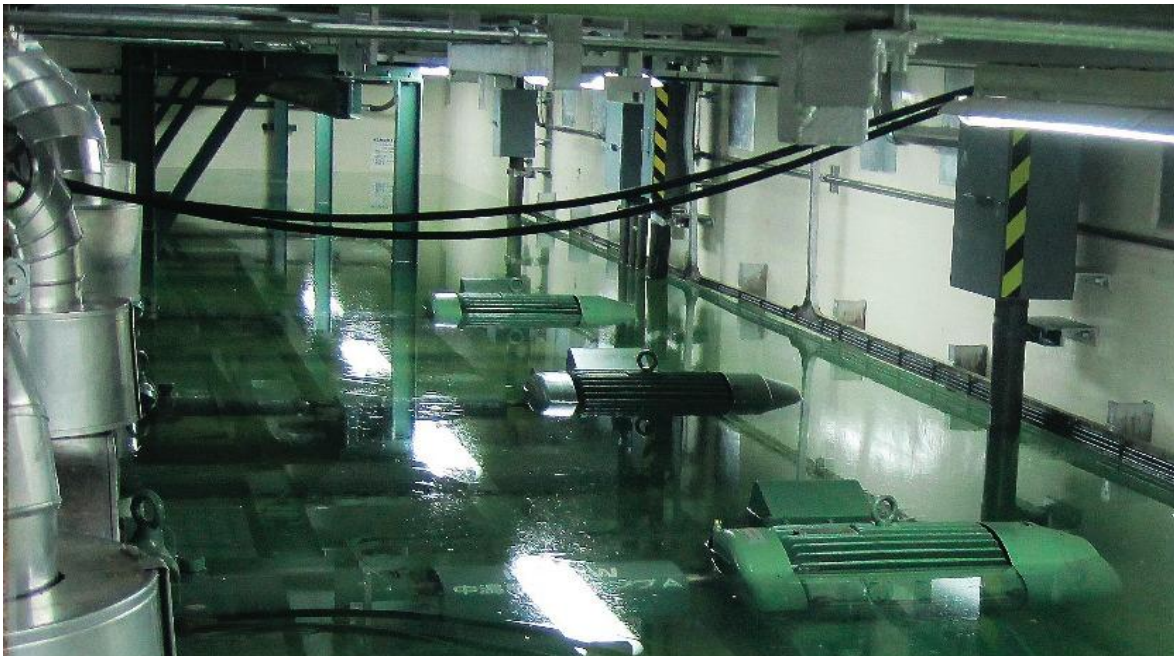
Figure 2. As a result of the insufficient flood design, this valuable equipment in reactor building three was rendered useless (Strickland, 2011).
