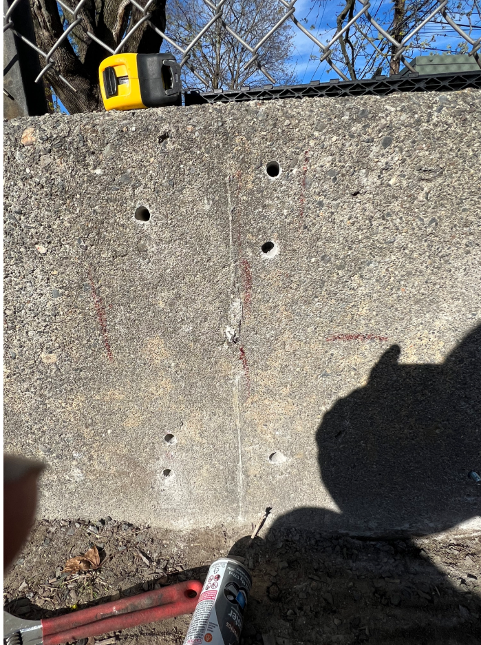
Figure 10: A Series of Failed Holes in YWCA CM Retaining Wall
