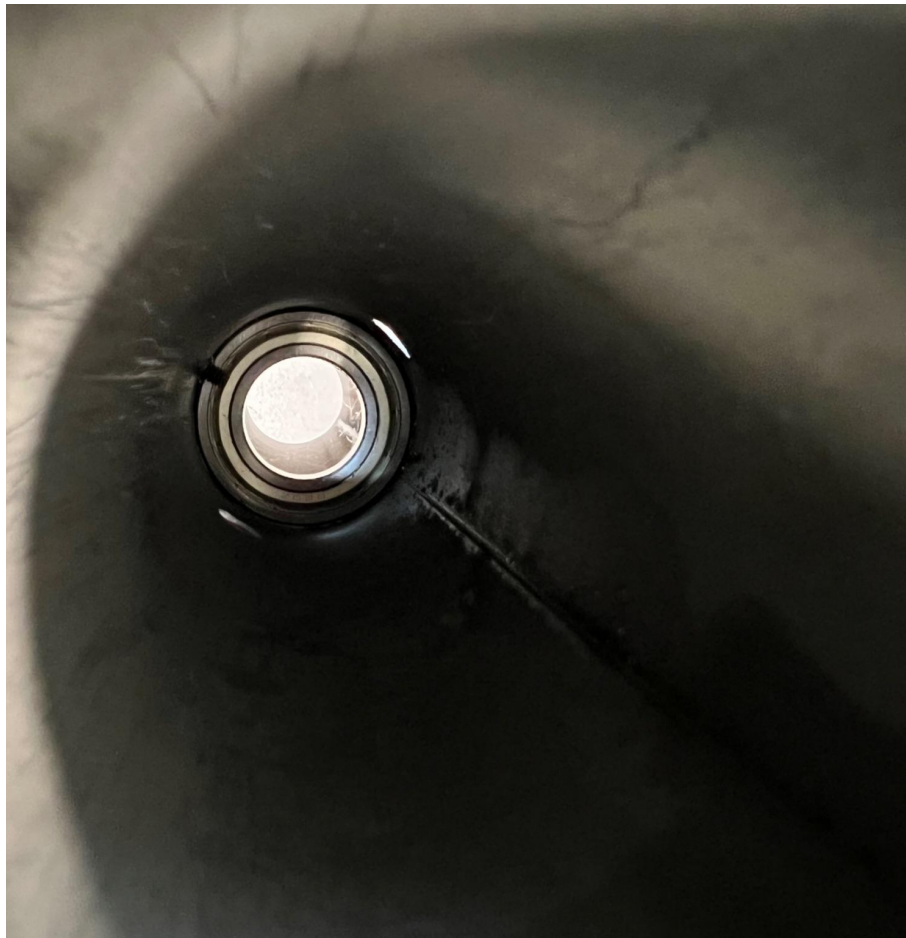
Image 5: Ball Bearing Inside of Blue Upper Section of Tower Crane
