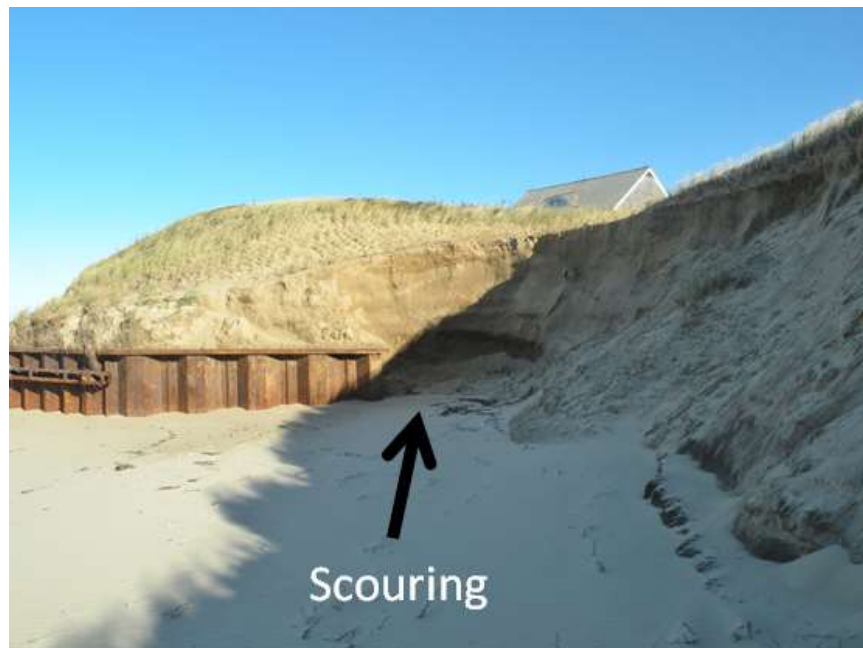
Figure 5: Seawall with Scouring on the Northwest Shore of Nantucket
