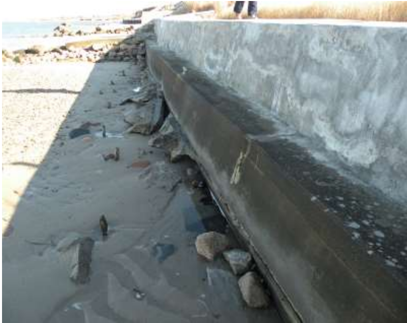
Figure 35: Vertical Scouring at Seawall, Quaise Road
