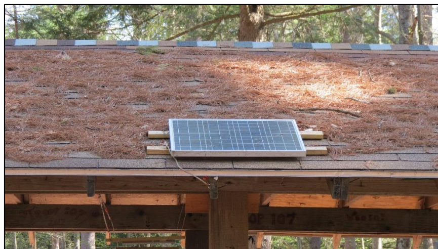
Figure 18 - PV panel roof-mounted on a hard shelter roof at TVSR
