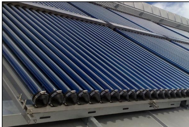
Figure 14 - A thermal solar panel installation [19].
