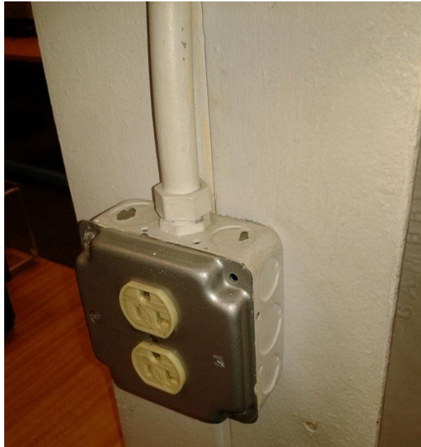
Figure 31: Two standard AC outlets, installed with the box exposed
