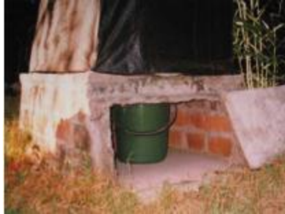
Figure 13. View from Behind Vault Showing Removed Access Slab, 20 L Collection Bucket within Vault, and Superstructure on Top Enclosing Toilet Pedestal for Privacy (Morgan, 2007)
