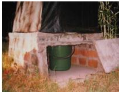
Figure 65. View of Collection Bucket for Feces within Vault after Removing Access Slab (Morgan, 2007)
