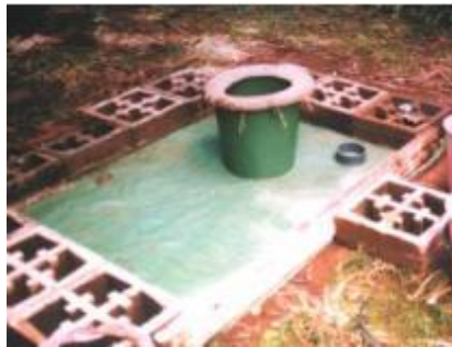
Figure 36. Brick Mould for Toilet Slab with Bucket and Metal Cylinder for Pedestal and Vent Pipe Space (Morgan, 2007)
