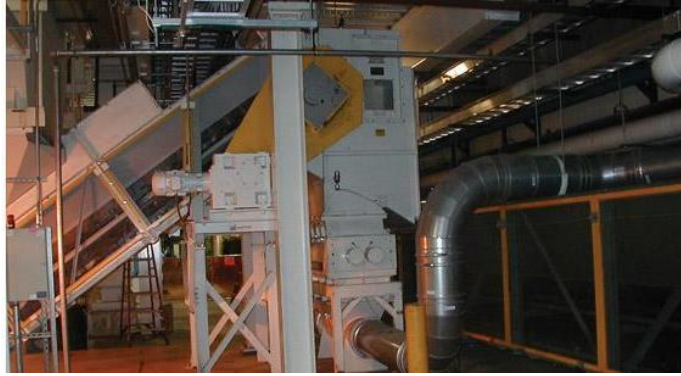
Fig. 3: Shredder Fed by a Conveyor and Connected to a Vacuum Tube [13].
