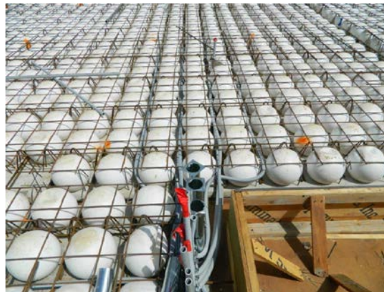
Figure 9: Integrated electrical system to the in the Bubbledeck before the onsite concrete is casted. *courtesy of Bubbledeck North America
