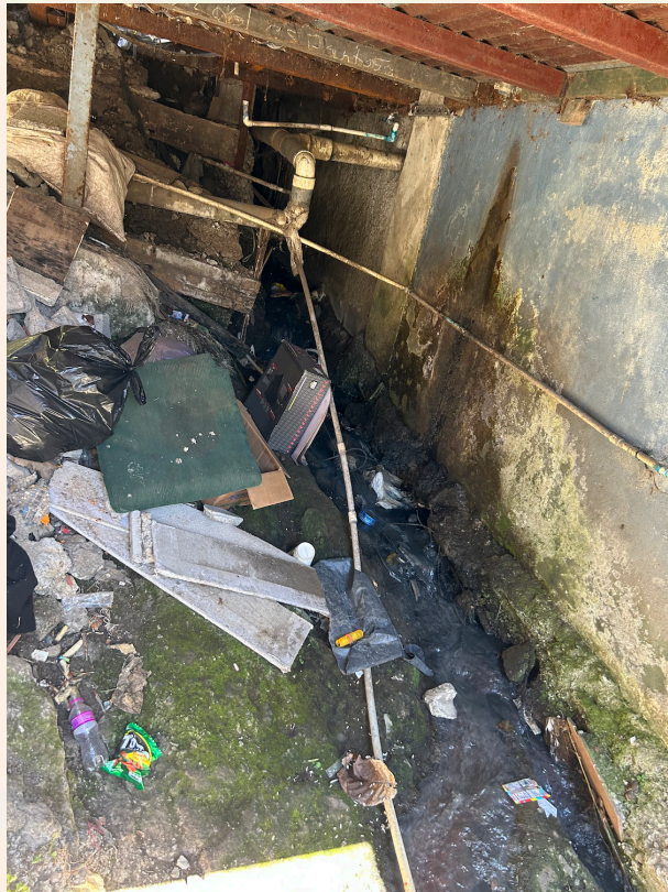
Figure 7: PVC Water Pipes attached to a home in La Carpio
