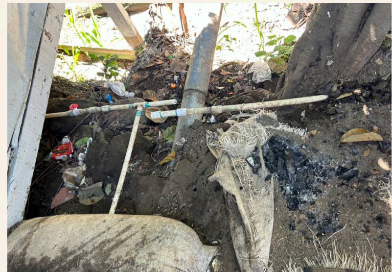
Figure 11: Broken Pipe located in Rio Torres
