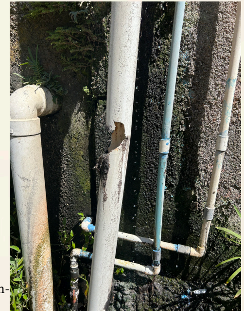
Figure 8: PVC Water Pipes in La Carpio
