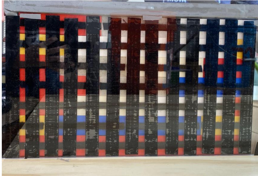
Figure 10: The backside of the watertightness roofing system showing the lattice pattern of Velcro
