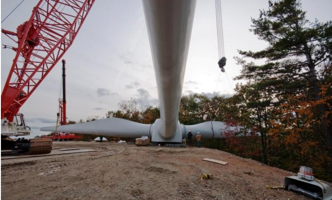
Figure 35: Shows the construction of a wind turbine rotor on a staging area in Princeton, MA
