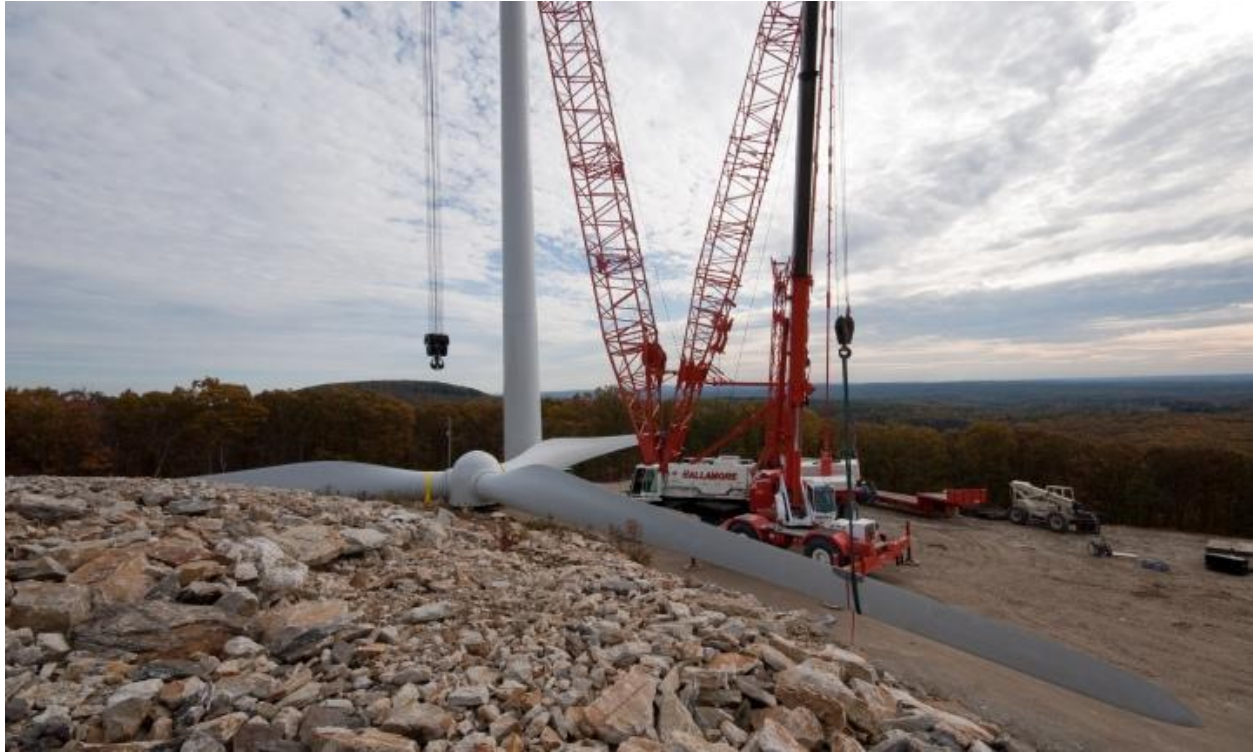
Figure 34: Shows the terrain of the staging areas at the Princeton wind farm, in Princeton, MA
