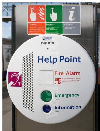
Figure 9: Example of a London Underground Help Point (London Particulars, 2011)
