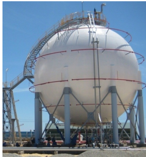
Figure 3.2 Example of a spherical tank for LPG [77]
