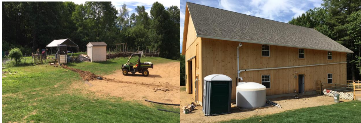
Figures 23 & 24: Construction Day 3: The Final Piping and Irrigation (left) and Collection and Storage (right) Image Source: Peter Mimeault
