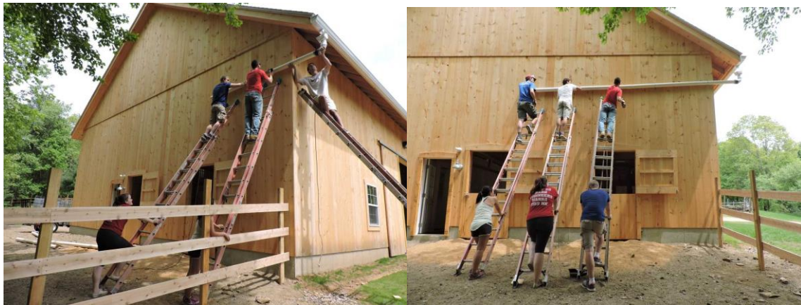
Figures 16 & 17: Construction Day 1: Beginning to Construct Collection Piping Image Source: Emilia Perez
