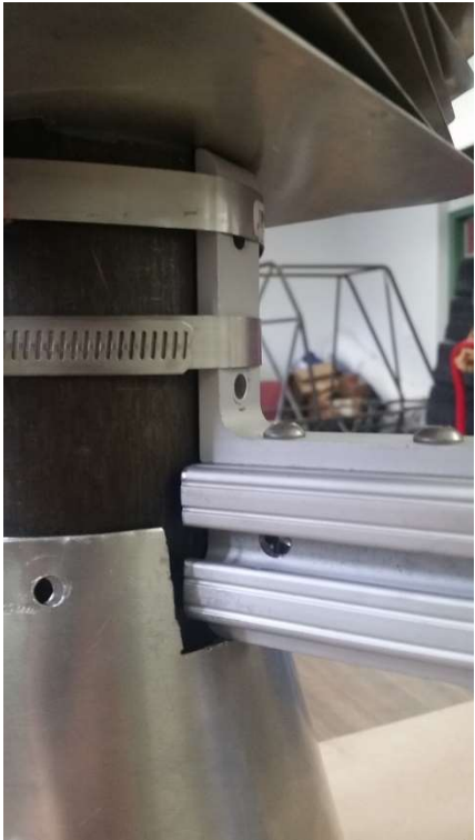
Figure 71- Close up view of Hose Clamps
