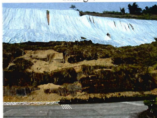
A minor landslide occurred next to campus. This retaining wall broke, but caused no other damage.
