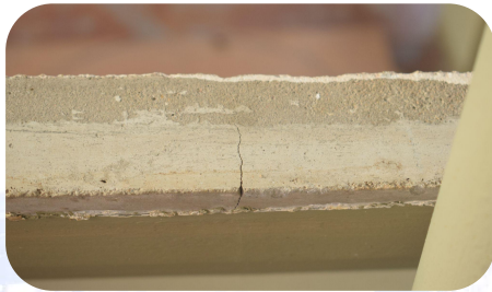
An unstable wood framework causes cracks in concrete
