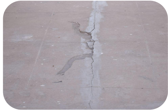
Cracks above the patched concrete layer
