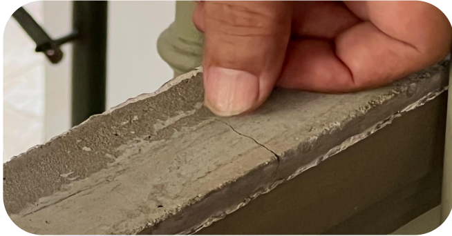
Small cracks in the middle between two edges
