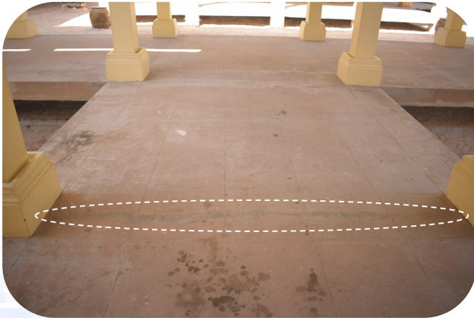
Cracks in the concrete walkways between two columns
