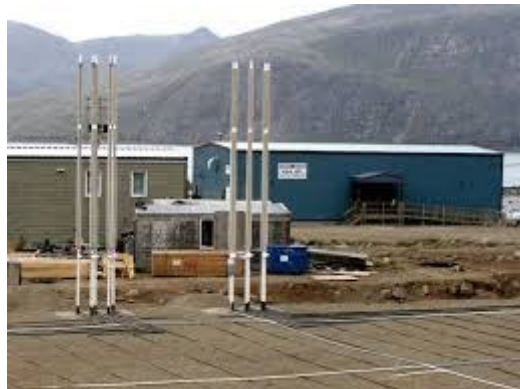
Figure 18: Thermosiphons used in building foundations
