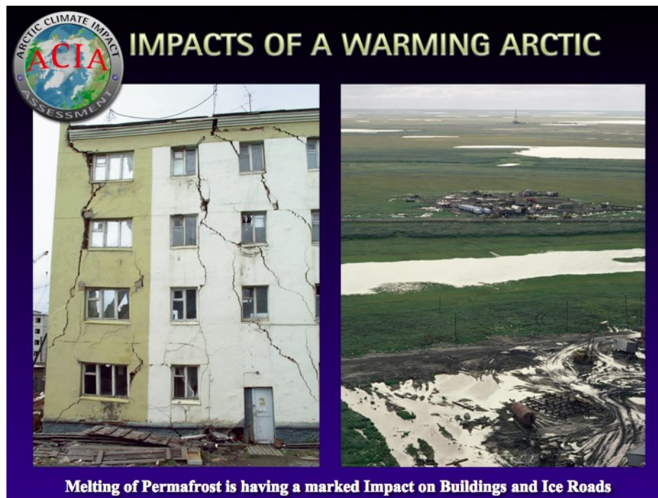
Figure 16: Structural damage caused by permafrost thaw
