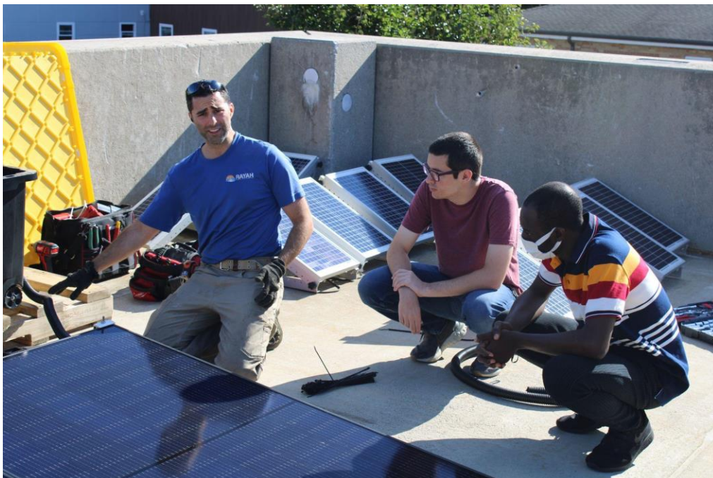
Figure 19. Displaying the installation of the PV array at the site on the top of the East Hall Parking garage. The installation expert, Tim Lewis, and Habebullah Adua are shown from left to right.
