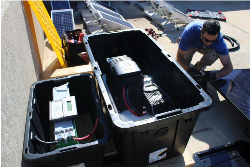
Figure 18. Displaying the installation of the PV array at the site on the top of the East Hall Parking garage. This is a close up of the weather proofing box containing the battery and the electronics.
