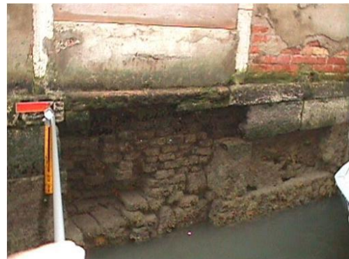
Figure 17: Canal Wall Damage
