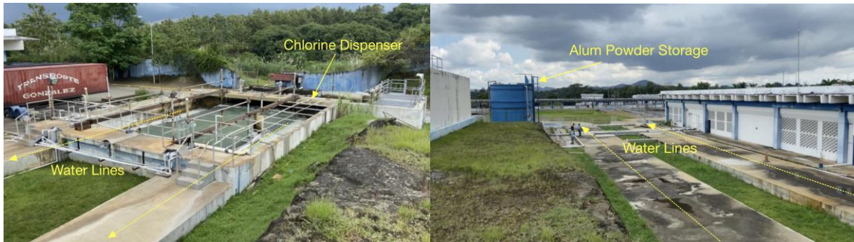
Figures 2.3-2.4. Water, piped from the reservoir, which is being mixed with chlorine and alum powder in the preliminary treatment steps. Chlorine is delivered through the labeled white PVC piping (left) and the water lines and Alum Powder storage tanks (right).
