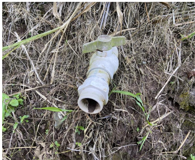
Figure 2.15. An input line for the tank trucks that deliver water on days where no water is available from the network. Upon closer inspection, it is uncapped and open to the elements with a pile of dirt easily visible from the outside.
