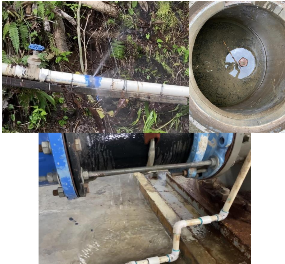
Figures 2.5-2.7. Examples of three leaks observed in the field: at Santa Librada Rural (left), at pump #1 in the Chivo Chivo pump station that services the Lucha Franco region just north of Santa Librada (middle), and a valve in Kuna Nega (right).
