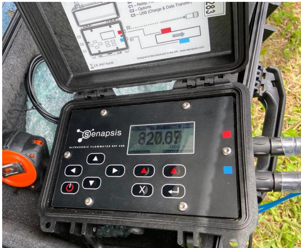
Figure 3.4. The flow meter reading device, displaying flow rate in gallons per minute (GPM).
