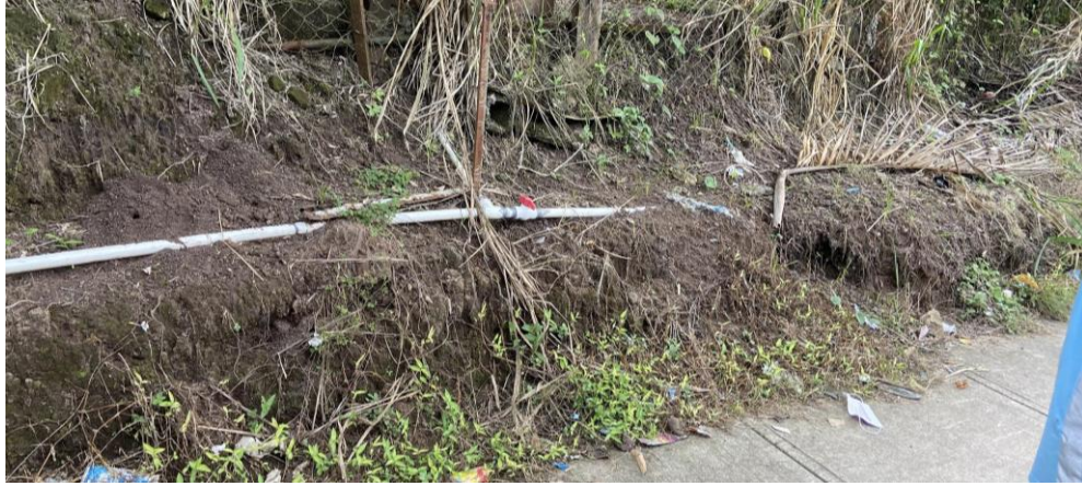
Figure 3.1. A pipe from which we gathered information, such as location, diameter, and material. We were able to walk alongside the main road to gather information about these pipes.
