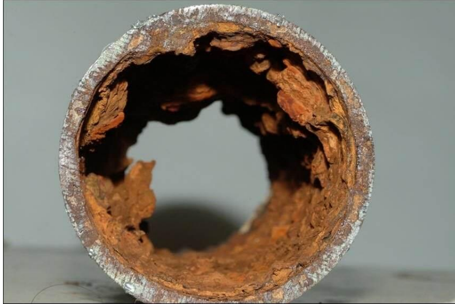
Figure 4.14. An example of a corroded cast iron pipe (“Corroded Cast Iron Pipe,” n.d.).
