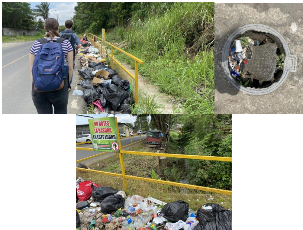
Figures 2.12-2.14. Examples of the degree to which garbage is present in these areas along the streets and in access points where it is in direct contact with aqueduct pipes.
