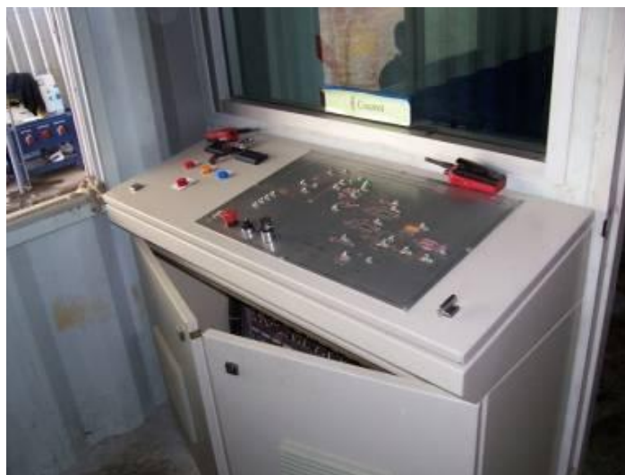
Figure 22: Control panel for processing system.
