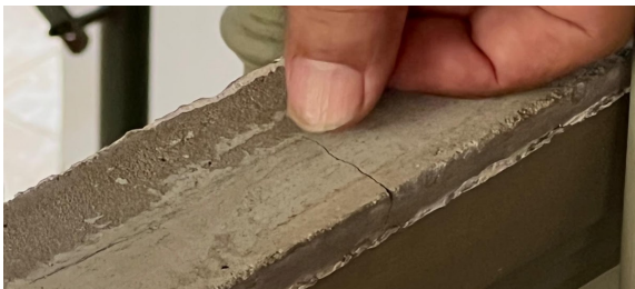
Figure 25. Concrete crack due to uneven weight distribution of wood framework
