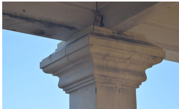
Figure 13. Cracks that form on the special design on top of a column
