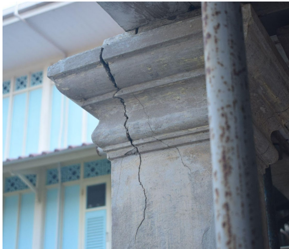
Figure 8. Examples of cracks in concrete columns at the Palace
