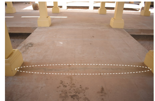
Figure 22. Cracks in the concrete walkway between two columns
