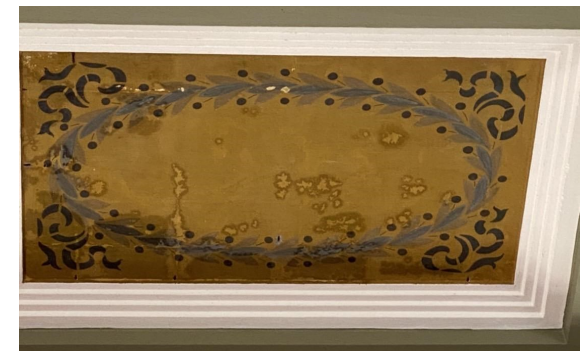
Figure 27. Pale marks with a droplet-like shape on the surface of a ceiling panel
