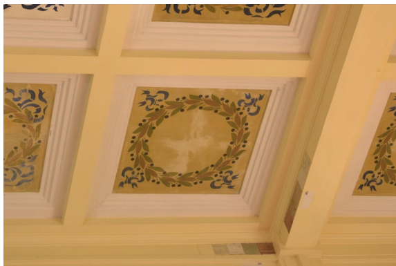
Figure 28. Plus sign marks with a yellow-like color due to rust on the steel rods
