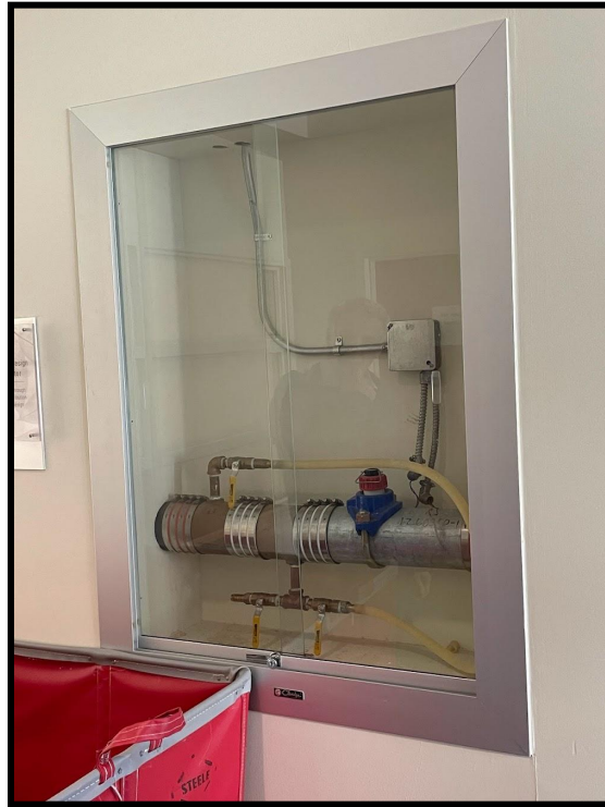
Figure 7. East Hall water sampling station in the lobby, April 2023
