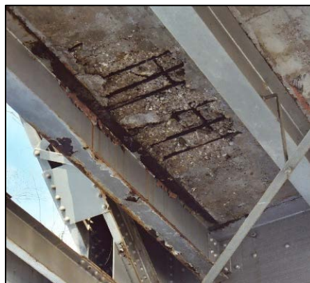
Figure 2: Corrosion of steel reinforcement on the bridge deck of the Devil's Elbow Bridge in Missouri [6].
