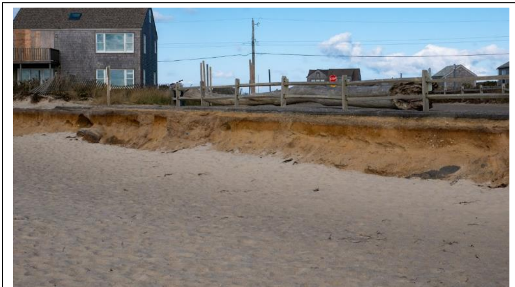
Figure 20: An example of the erosion at the Madaket Beach parking plot. The photo was captured during high tide.
