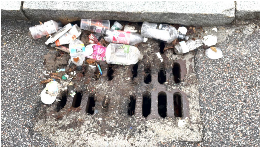
Figure 2: Image of Catch Basin with Litter
