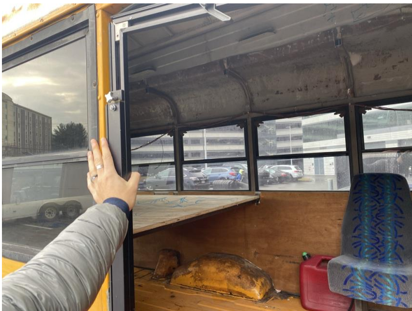
Figure 6, blower door frame
