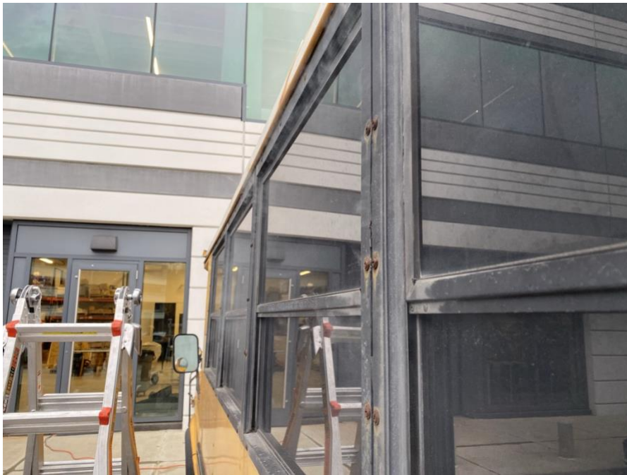
Figure 11, Fog positive pressure testing. The fog appears faint but was clear in person.
