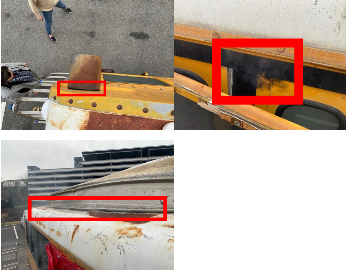
Figure 16, detailed photos of air leakage
