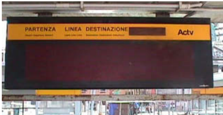
Figure 47. Non-functioning Electronic Sign.
