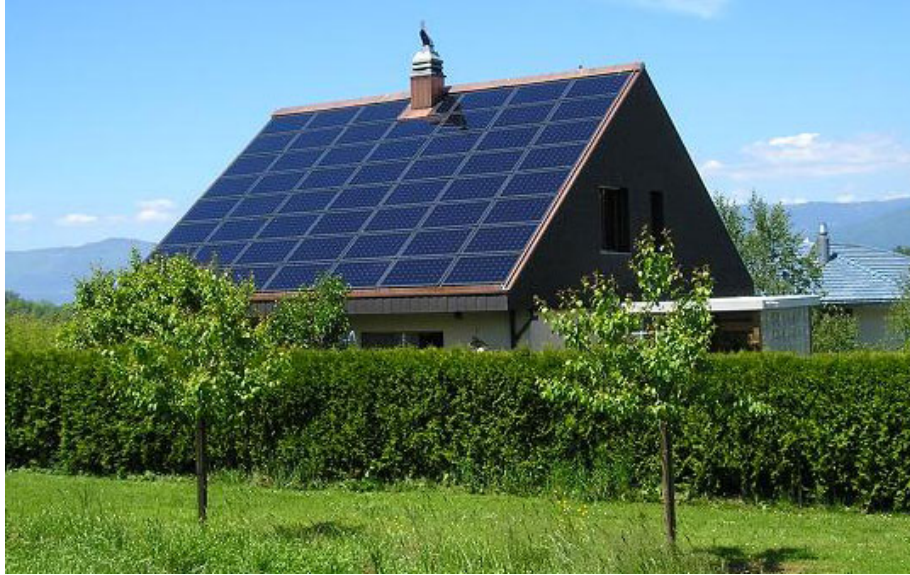
Figure 2.13: Domestic Photovoltaic Solar Panels
