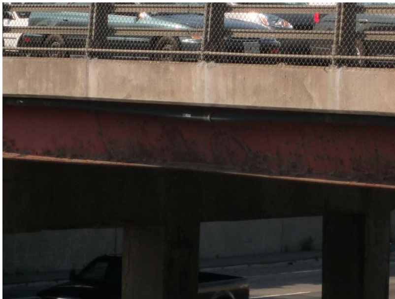
Figure 13: Bent girder from impact of collision
