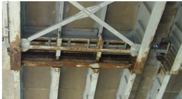
Figure 25: Example of corrosion on steel lateral bracing of bridge superstructure (taken from http://minnesota.publicradio.org/collections/special/columns/news_cut )
