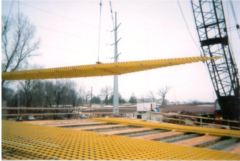
Figure 57: Polymer grid system being laid into bridge deck by a crane (taken from http://www.engr.wisc.edu )
