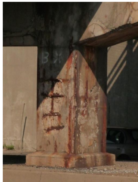
Figure 26: Heavily corroded reinforced concrete support on the Belmont Street/Route 9 Bridge
