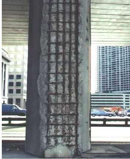
Figure 21: Exposed steel rebar in reinforced concrete column (taken from http://www.corrosion-club.com )
