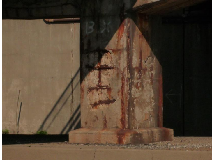
Figure 14: Extensive column corrosion on Belmont Street/Route 9 Bridge
