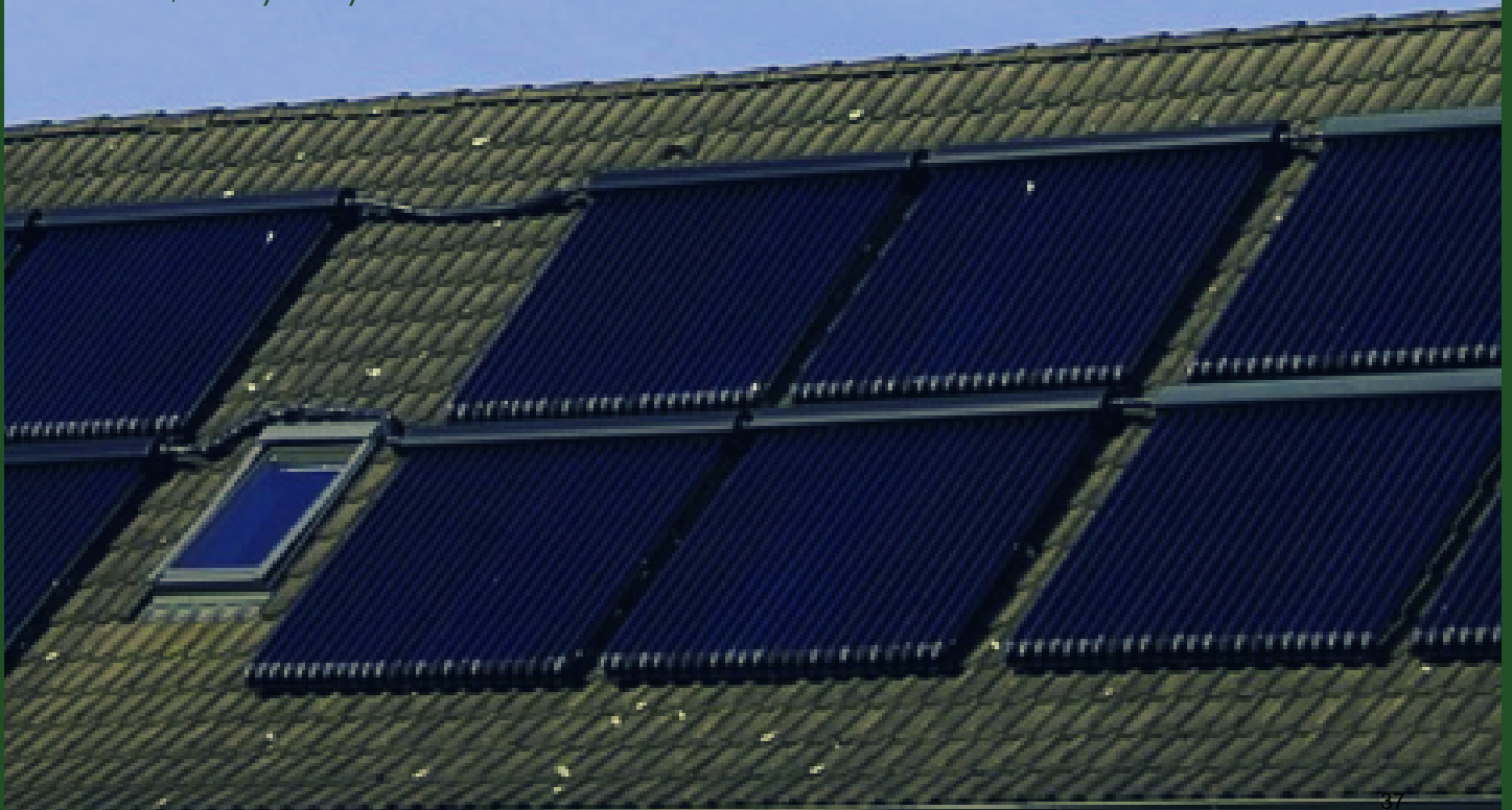
Figure 35: Solar panels on a roof
